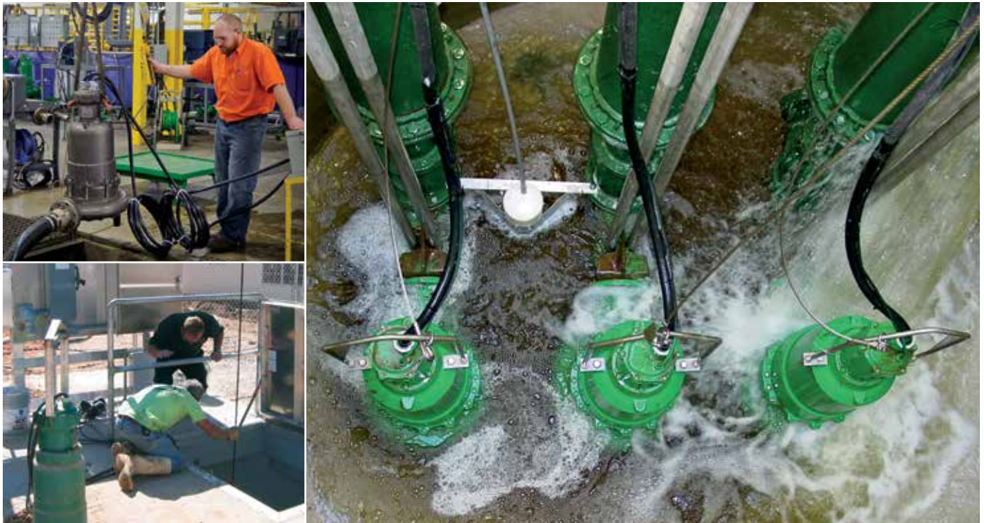
Pictured at top left: Certified CSA test lab. Pictured at bottom left: A submersible solids handling pump being installed into a lift station for a new apartment complex. Pictured at right: Three Hydromatic SBL pumps installed in Jefferson Parish, LA.
