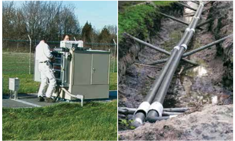
Pictured at left: Below-grade installation also shows electrical control console. Pictured at right: In-ground piping installation in progress.
